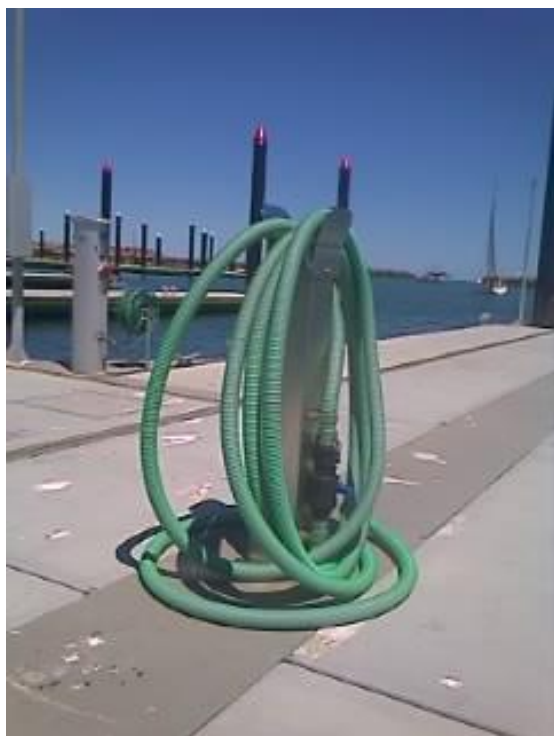
Figure 1: The CYCSA vacuum effluent disposal facility at Marina West
