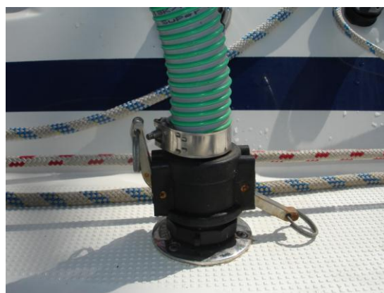
Figure 3: Pumpout hose connected to deck fitting via Camlock Coupling
